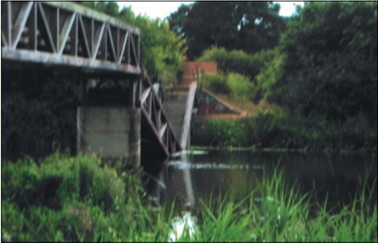
The collapsed Ashford Lane footbridge over the Jubilee River.
