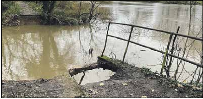
The collapsed section of the towpath.
