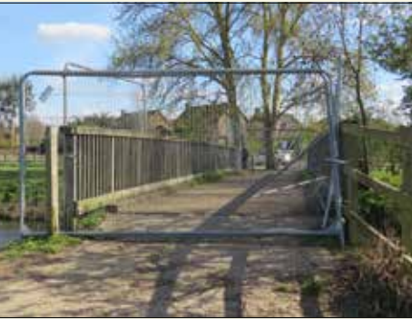
Kempston Mill Bridge awaiting repairs. Photo: Barry Ingram
