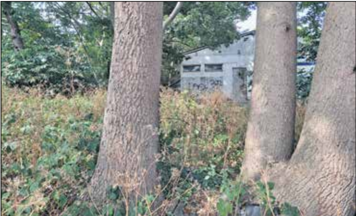
The deteriorating scout hut. Photo: Des Garrahan.
